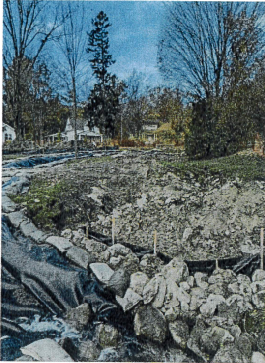
Photo 1. Looking upstream from alley at former water wheel location and relocated channel.
