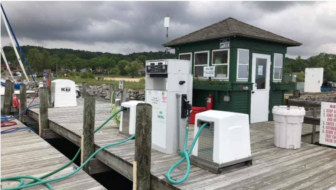
Figure 12: Service pier, fuel dispensers, sanitary pumpout
