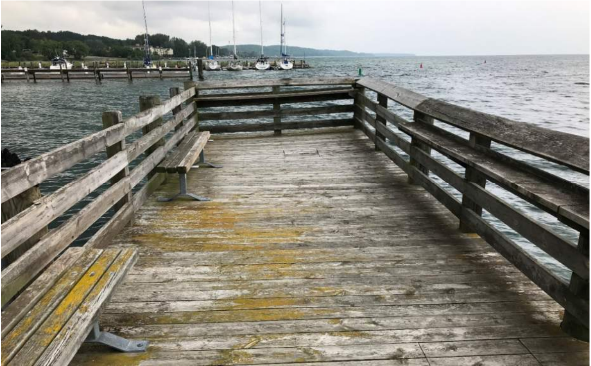
Figure 19: Fishing pier; note lack of ADA-compliant rail; note uneven deck/rail
