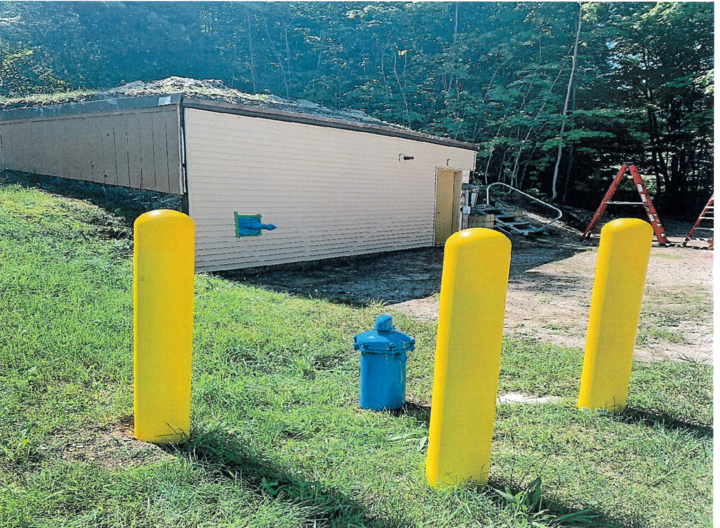
Top: Exterior wall degradation as discussed last month compounded by an infestation of small woodland creatures.
