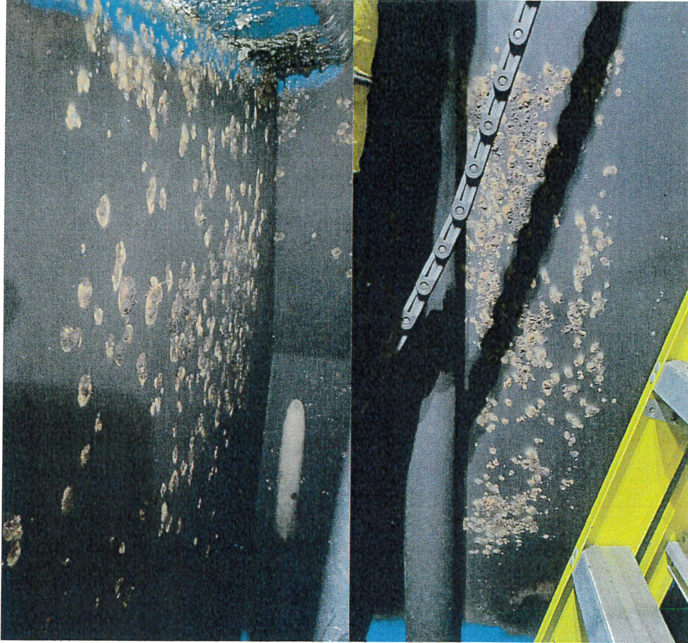
Tank wall pitting
