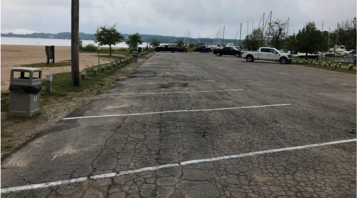
Figure 6: Representative photo of main parking lot condition; note cracking and elevation relative to beach
