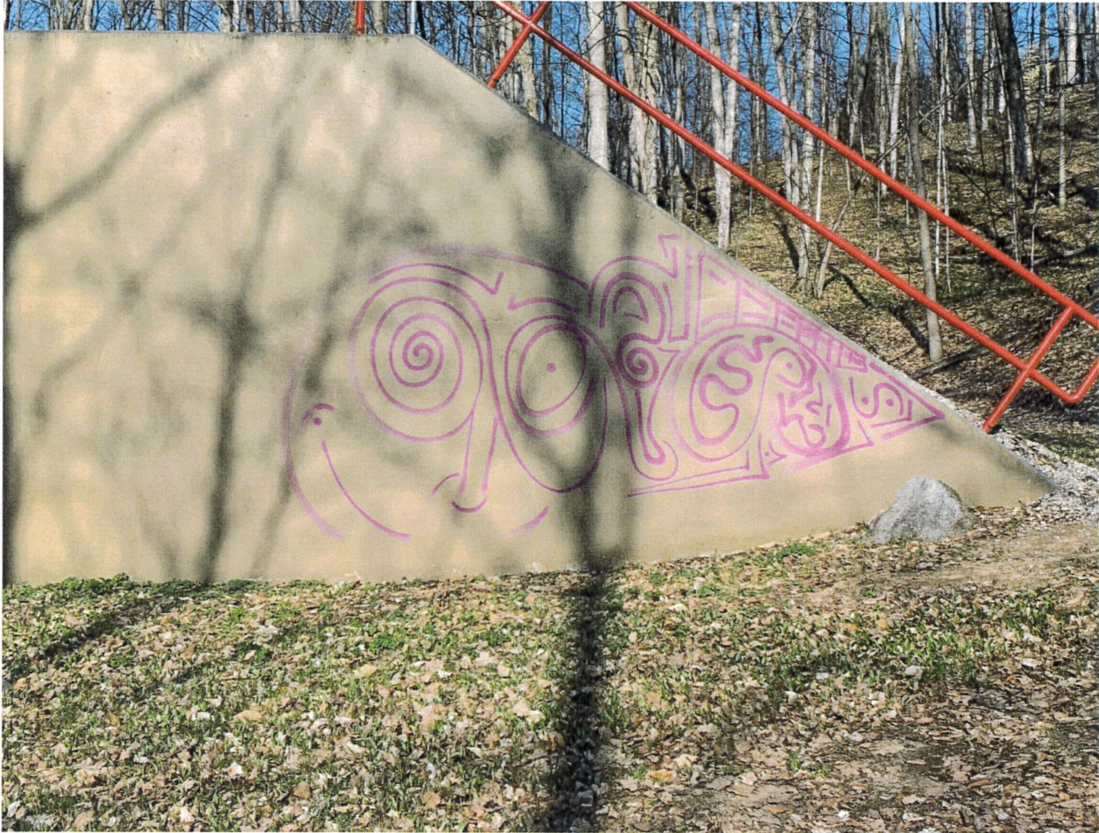
Attachment C; Graffiti at the Ground Storage Tank
