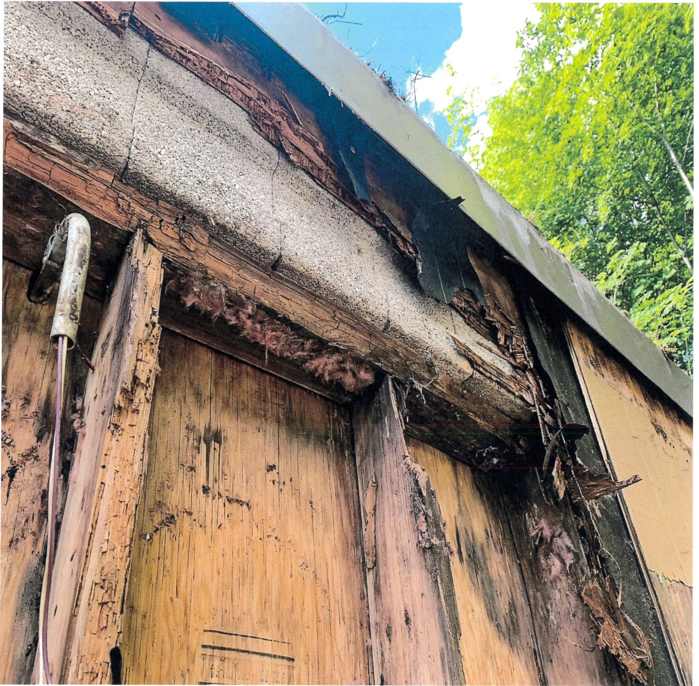
View of rotten wood wall at the concrete ceiling.
