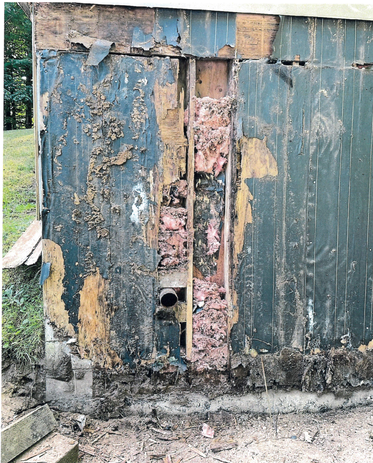
Water damage to exterior wall, mice nests in insulation. Wood completely rotted.
